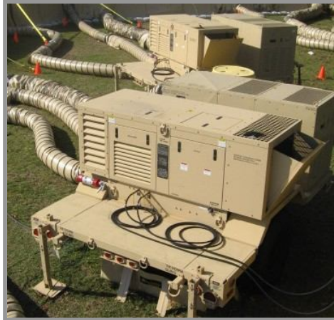
The Standard USMC COC GETT – 10Ton ECU with 23kW Generator
